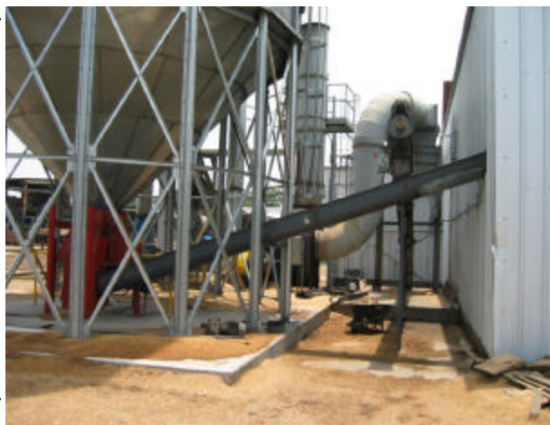
Shown above is a metal bin with a Flying Dutchman unloader and exit auger burning green fuel at a sawmill installation.
